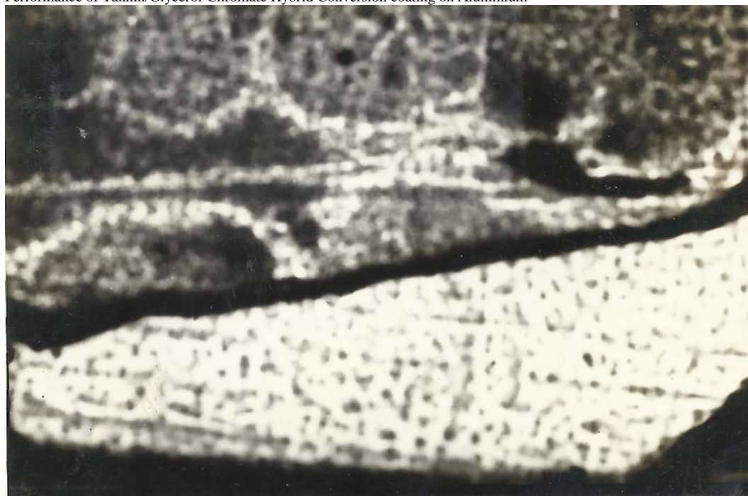
Figure 2. Optical photograph of lacquer coated aluminium specimen after exposure to high humidity for 255 hours showing paint delamination and incipient pitting corrosion at the edge of a pre-scratched region where lacquer had been lifted up as a result of paint delamination. \times 1000 .
