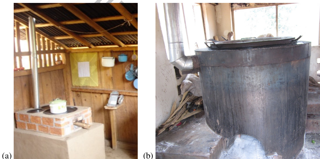
Fig. 2. Examples of cookstoves with chimney stacks: (a) rural dwelling in Mexico; (b) institutional stove at a prison's facility in Uganda. (Photographs courtesy of Dr Omar Masera-Cerutti from Instituto de Investigaciones en Ecosistemas y Sustentabilidad, CP)
