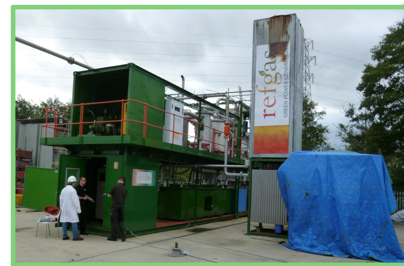
Figure 2. Refgas gasification plant, Chester, UK
