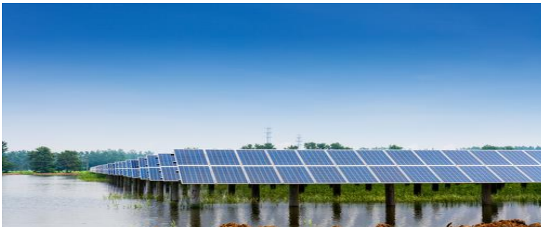
Figure 2.3. Installed solar modules. [10]
