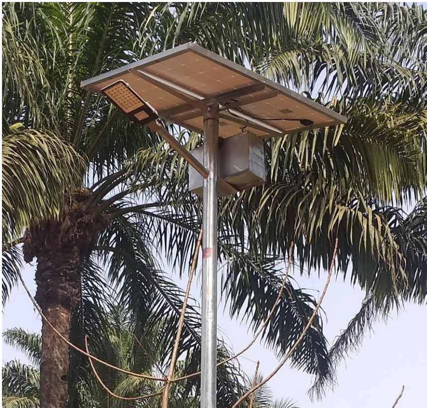
Figure 6.1. A stand-alone street lighting system.
