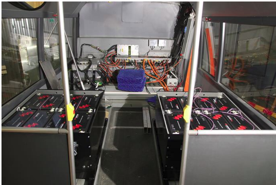
Figure 44. Leclanché LTO battery packs at the rear cabin (VTT, 2016)
