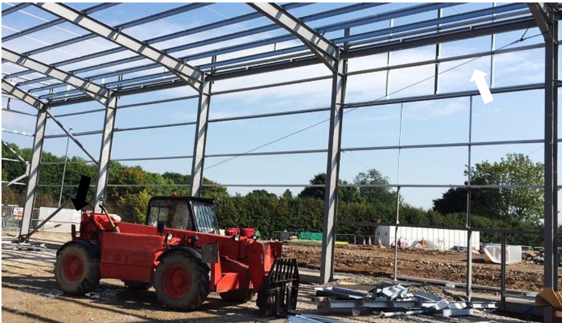
Figure 4-49. A portable manual hoist along with maxiflex wire rope being used to pull the steel frame to an acceptable position and orientation
