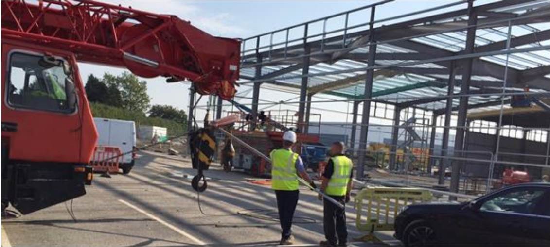
Figure 4-43. The position of the crane to erect the second side of the building
