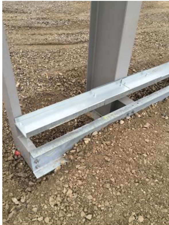
Figure 4-36. Backfilled outer side of the steelwork with gravel to avoid movement due to pouring concrete
