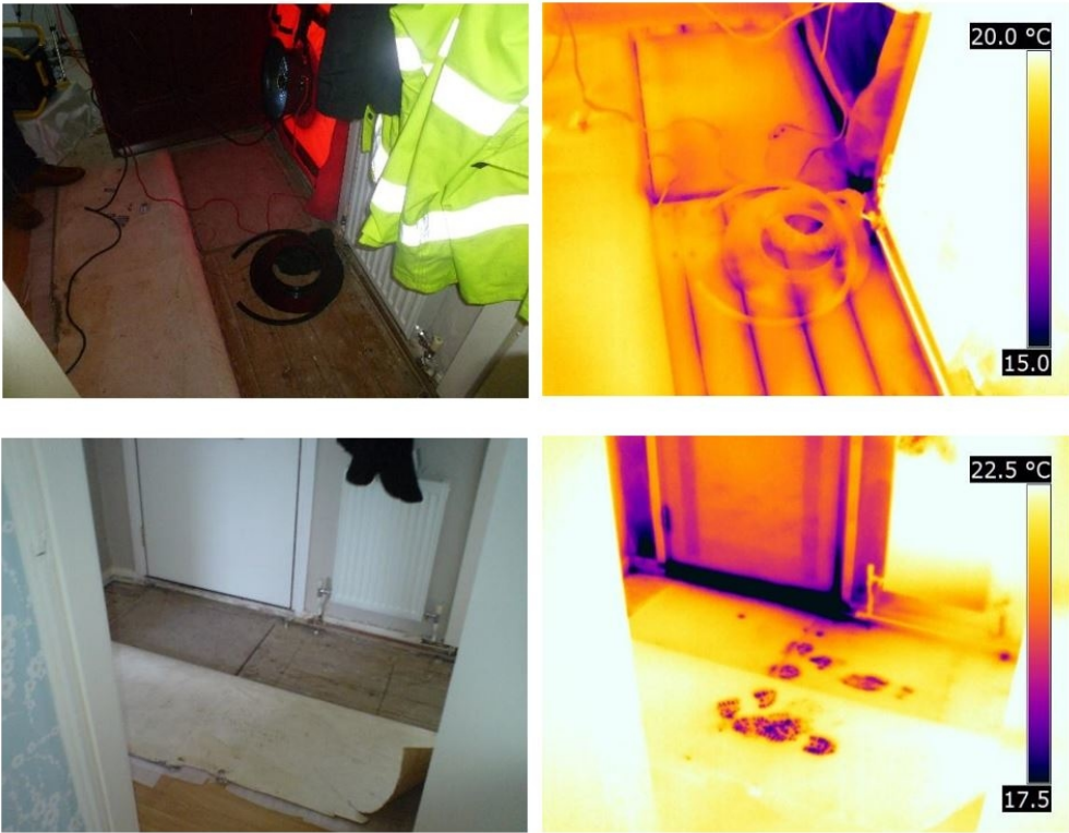
Figure 7, Infiltration through hallway floor pre retrofit (top) and post retrofit (bottom) 203x158mm (120 x 120 DPI)
