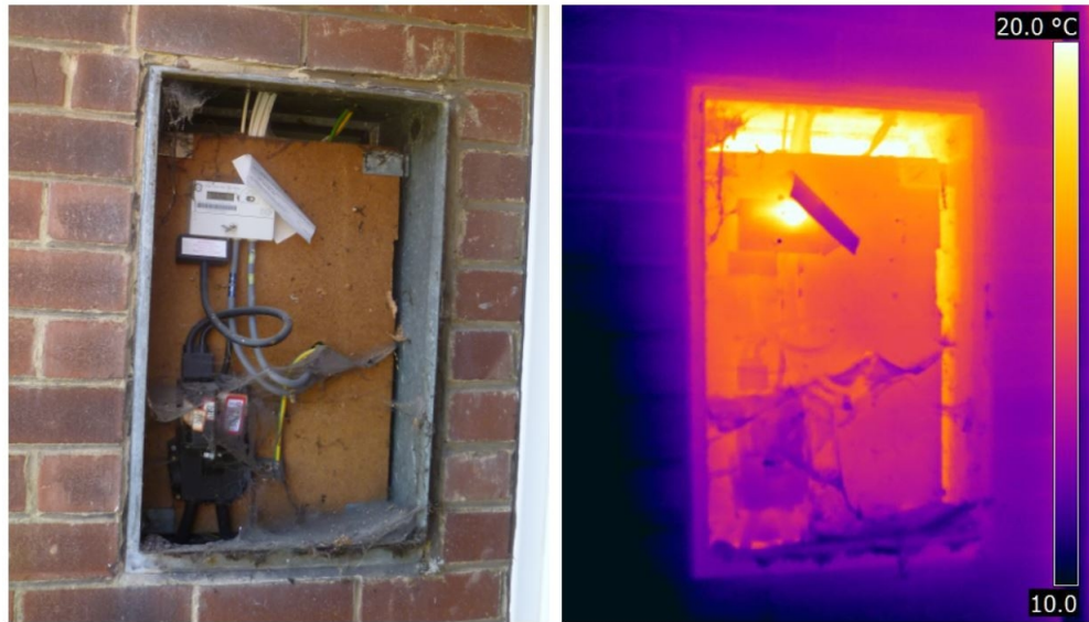
Figure 6, Exfiltration through unsealed electricity meter open to interior of dwelling
