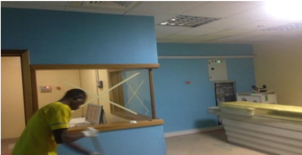
Plate 8: The operator control room with lead glass in the 16 slice CT room.
