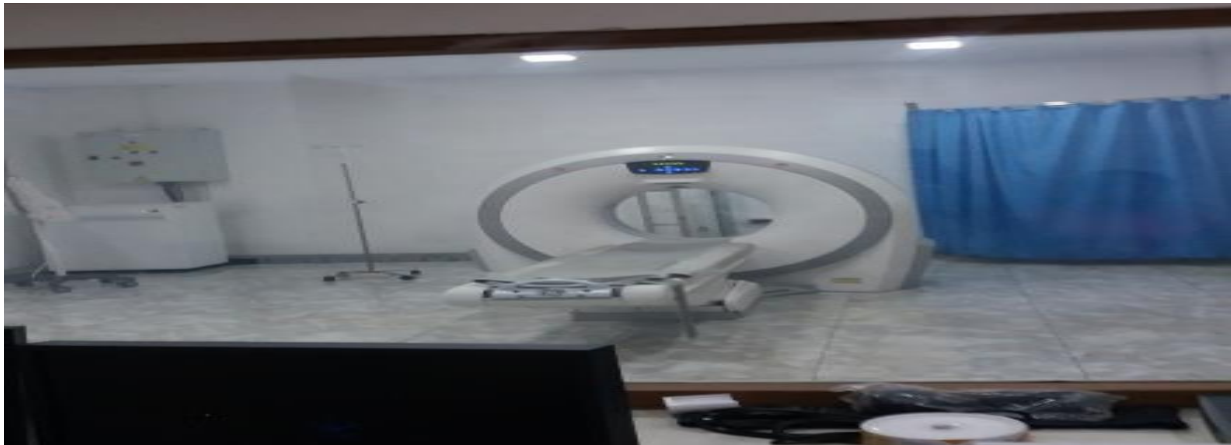
Plate 13: The 16-slice CT through the lead glass from the operator's area.
