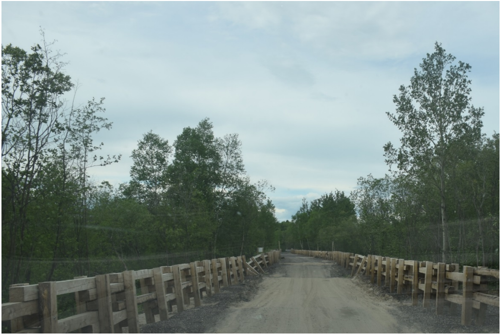
Appendix 1: Photo 7- The fence along the road to Birch Island with damage from the May flooding
