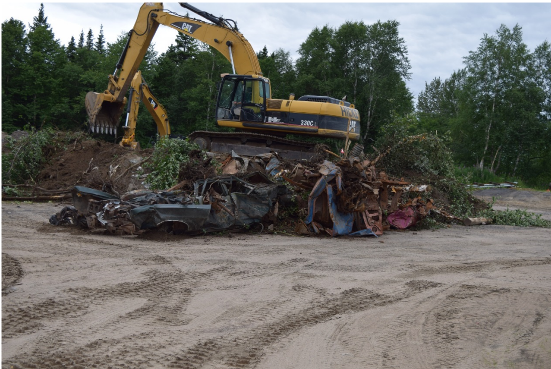
Appendix 1: Photo 60- Old car being pulled out of the creek that was most likely put there for bank stabilization HWL
