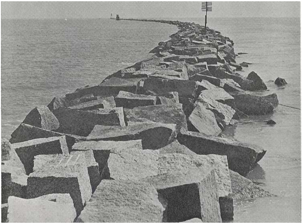
FIG. 4. Jetty at Galveston, Texas. Built with Precambrian granite blocks quarried and shipped from the Central Mineral Region (Pl. I). (Photograph by Corps of Engineers, U. S. Army, Galveston District, Galveston, Texas.)
