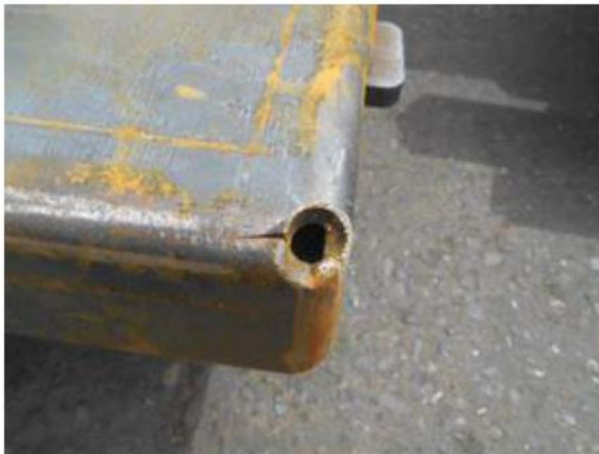
Figure 5 Weld cracking initiated from a small cut-out intended to avoid the problem of intersecting welds in fabrication of a hollow section.
