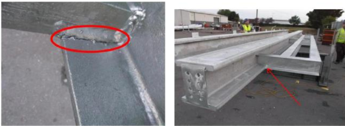
Figure 7 Cracking at the highly constrained joint between a smaller sub-assembly and a large I-beam. Separate fabrication of the two components and subsequent bolting would have eliminated the problem.
