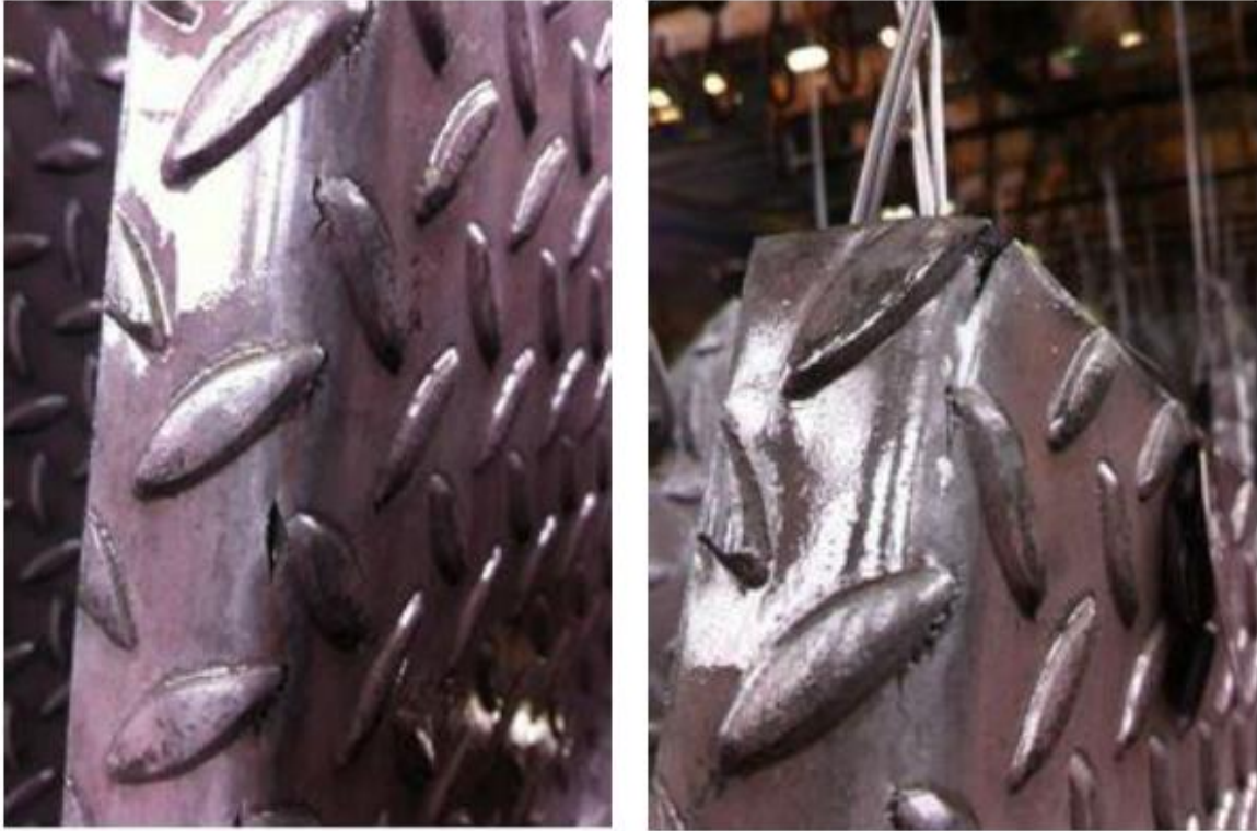
Figure 4 The cracking seen here is due to the steel checker plate having too tight a bend radius.
