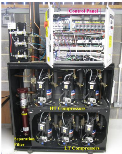
(a) Pack of Compressors
