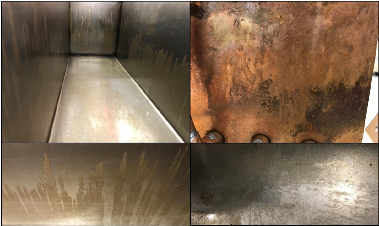
561 562 Figure 13: Pitting on the surface of the mild steel container and copper fins
