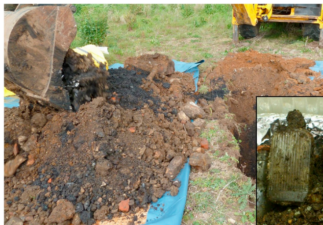
Fig. 2. Waste extracted from Leigh Marshes trial pit 6 included a sealed poison bottle containing an unidentified liquid (insert).
