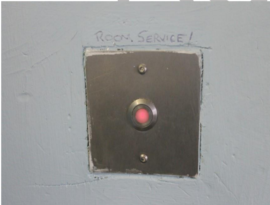
Fig 4. Emergency alarm 'Room Service' graffiti (Image: Roz Currie)
