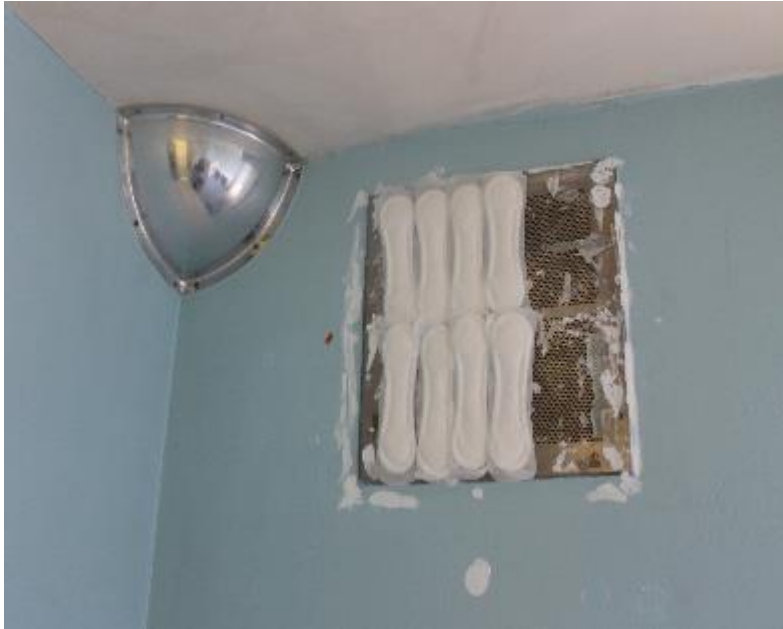
Fig. 3 Sanitary towels covering air vent – (Image: Roz Currie)
