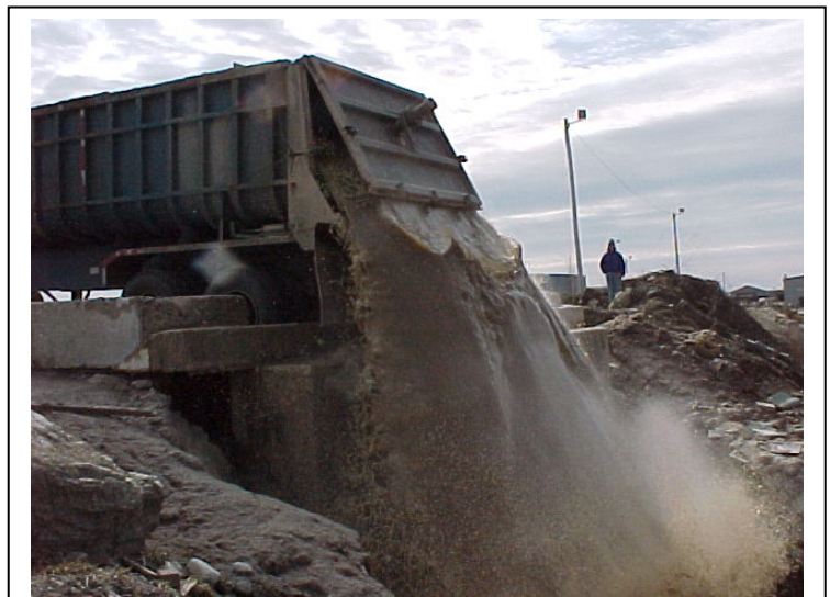
Sludge being dumped into the Rockland Quarry
