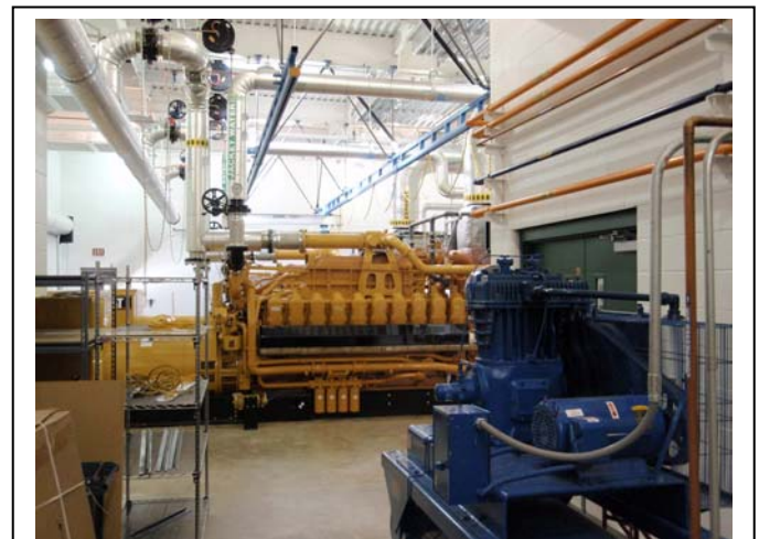
Landfill Gas Combustor, Crossroads Landfill Norridgewock, Maine 2009
