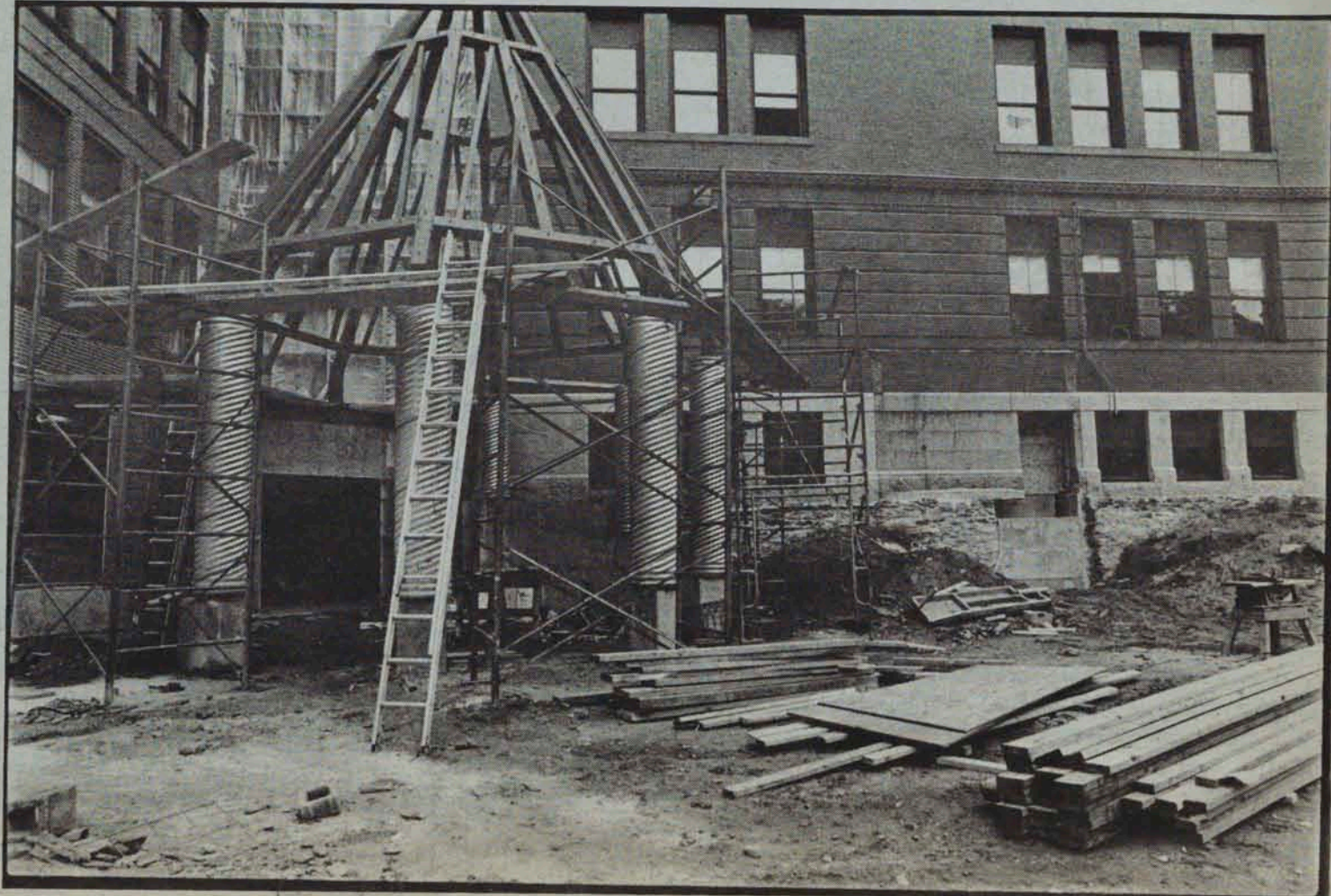
What are we trying to build here? Lincoln Middle School isn't the only confusing mess in school construction. FILE PHOTO/SHOSHANNAH WHITE
