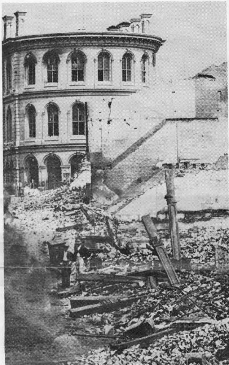
THE CUSTOMS HOUSE at Middle and Exchange Streets was one of the few major buildings to survive. The fire weakened it structurally, however, and it had to be taken down.
