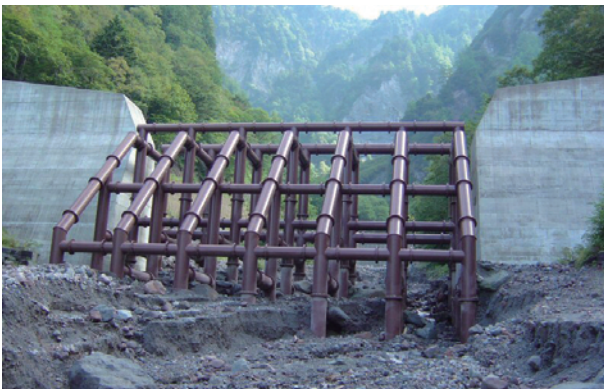
Figure 9 : Open Type Check Dam Made from Steel Pipes Source: Reference [27]
