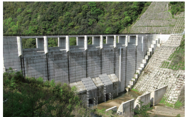
Figure 10 : Open Type Dam to Control Flooding (upper side of a dam) Source: Reference [28]
