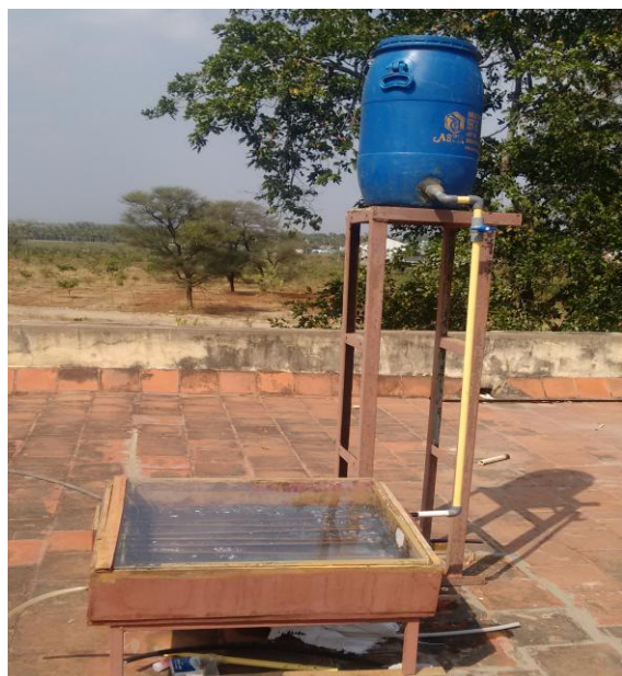
Figure: 2 Solar water heater
