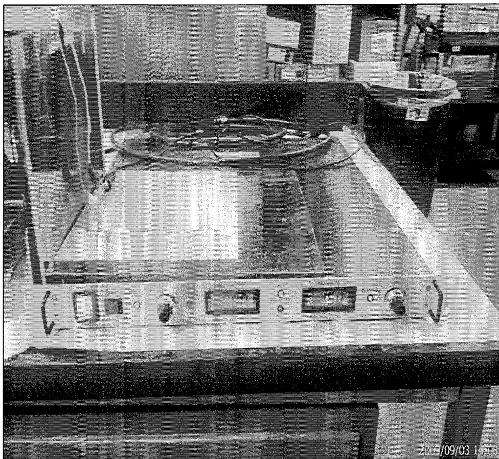
Figure 3.6 High Voltage Electricity Source (Located at CTH).
