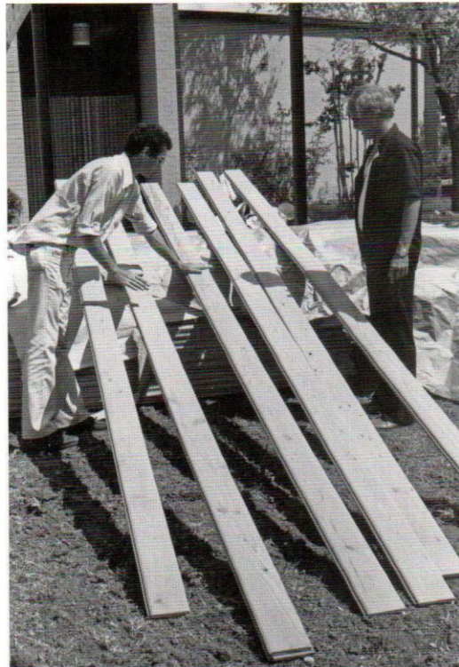
Lyle Novinski and Father Fischer lay out planks for the ceiling of Lynch porch where Sunday liturgies were held until the Church of the Incarnation was completed in 1985.
