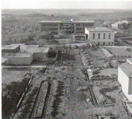
Braniff Mall under construction in 1967, with Braniff Building, Tower, and Gorman Lecture Center complete.
