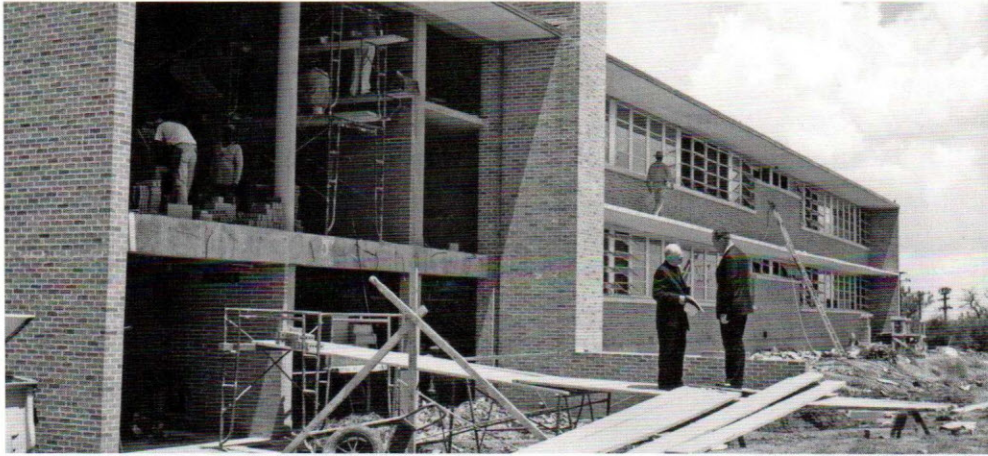
Marian Hall under construction, 1956. In 1973 the dormitory was renamed in honor of the late Sister Mary Margaret O'Connell, ssmn, the first Registrar.
