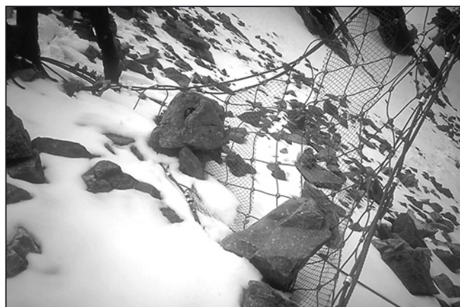
Snow-nets retaining rocks in summer. In winter the nets prevent the triggering of avalanches. Photo: Marcia Philips.
