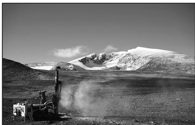
Drilling a 9 m deep borehole in permafrost on Dovrefjell, October 2001. Photo: Ketil Isaksen
