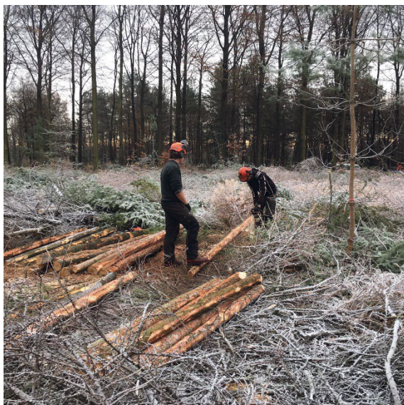
Figure 3: Posts for an enclosure being built by HELICON students during a practical. (Photo M. Marsman).
