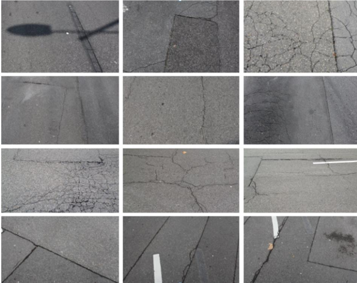
Figure 66. 12 image samples including linear, block and alligator (fatigue) cracks (Miraliakbari, et al., 2016)
