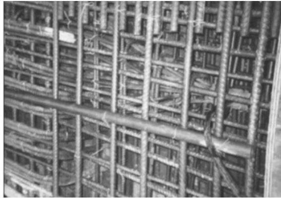
Figure 12: An example of congested reinforcement: an ideal application for SCC [17].
