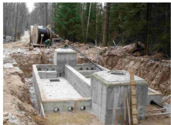
Figure 5: Concrete joint bay. Picture: Vattenfall
