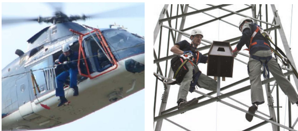
Figure 62: Installation of bird protection devices on a transmission line per helicopter (left, picture: RWE). Nesting aid installation on a transmission pylon (right).
