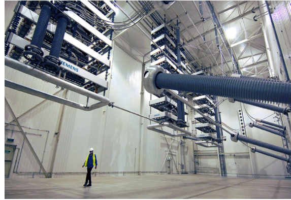
Figure 44: HVDC converter station. Picture: Siemens.
