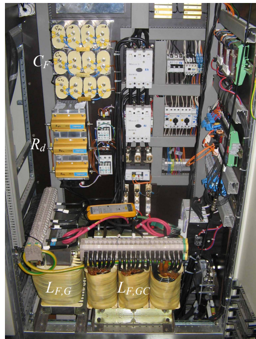
Fig. 4-49 A picture of the LCL-filter of the test bench; L_{F,G} : grid side inductor, L_{F,GC} : inductor of the grid side converter; C_F : filter capacitor; R_d : resistor for passive damping
