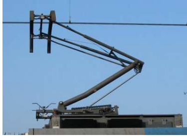
Figure 1.1.: Overhead Cable with a Current Collector
