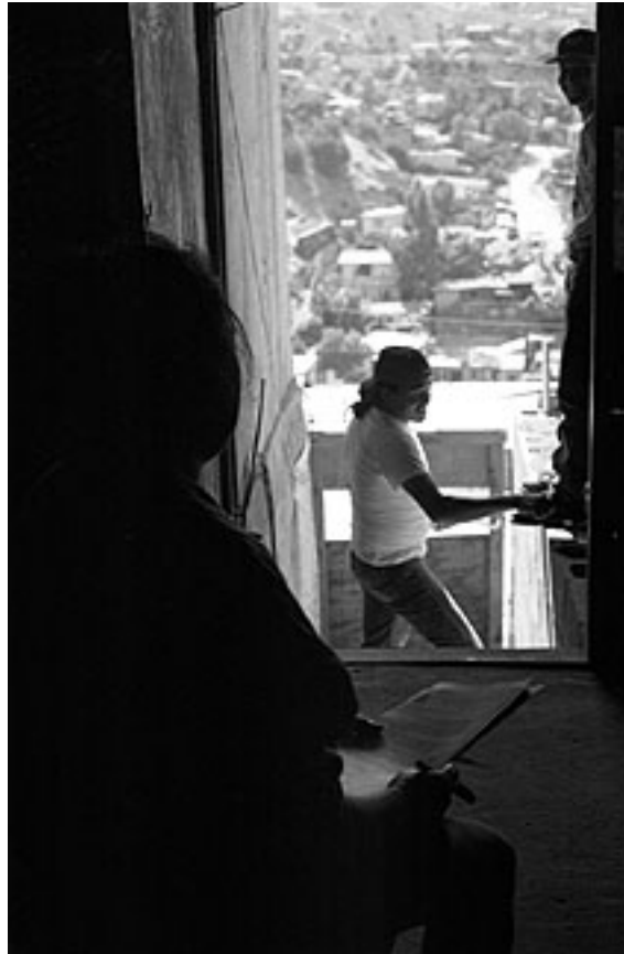
Figure 15: A room in Delfina's house, under construction. Photo by Luz Aida Ruiz Martinez, Grupo Factor X
