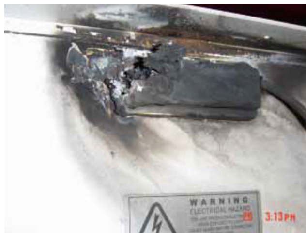
Fig. 7 Junction box failure caused by arcing. 4
