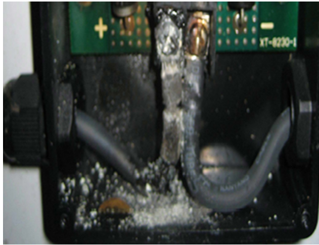
Fig. 8 Junction box failure. Courtesy: John Wohlgemuth, NREL.
