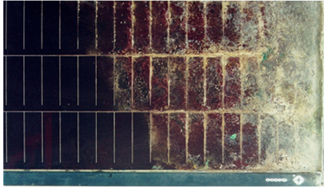
Fig. 1 Bar graph-type degradation caused by moisture ingress and corrosion; inward and sideways.
