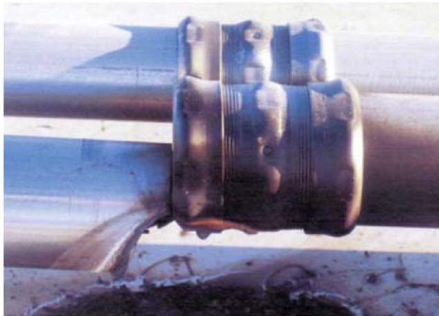
Fig. 13 The failure of an improperly specified and installed expansion joint possibly triggered the Bakersfield fire. 9 However, this was not the first fault in the system.
