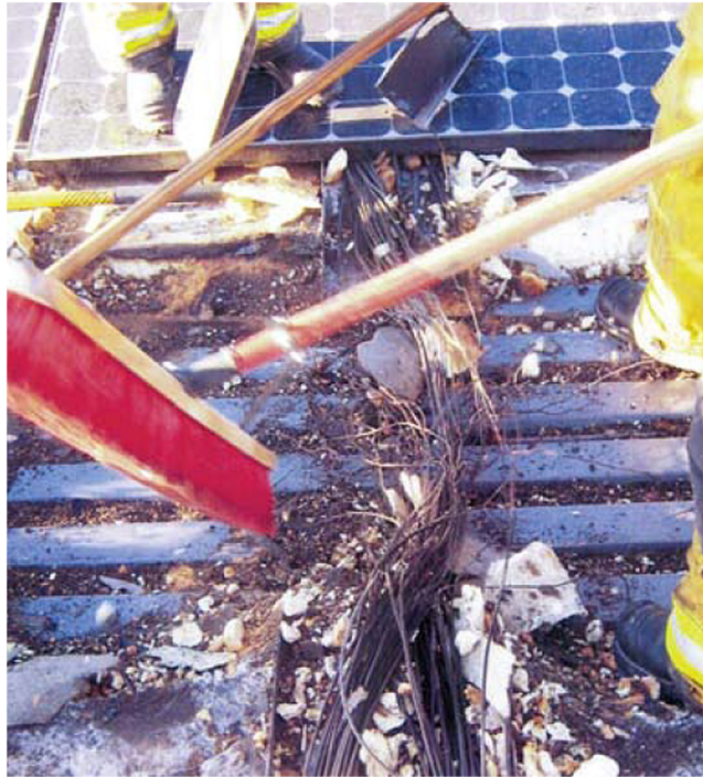
Fig. 14 The possibility of an undetected first fault in PV source-circuit conductors highlights the importance of proper commissioning procedures and improved wire management practices throughout the industry. 9
