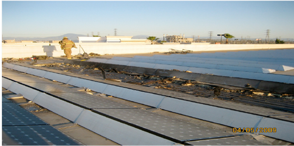
Fig. 12 PV arcing and fire in Target store at Bakersfield, CA.
