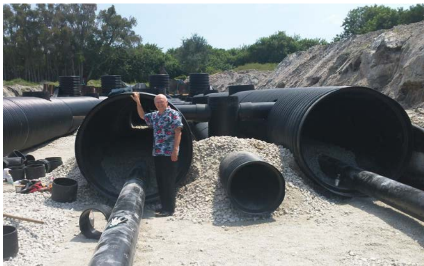
Figure 39. Up-Flow Filter in a Pipe
