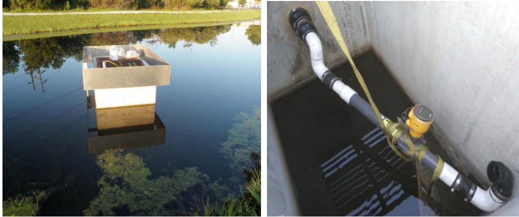
Figure 34: Outlet structure and the flow meter unit inside
