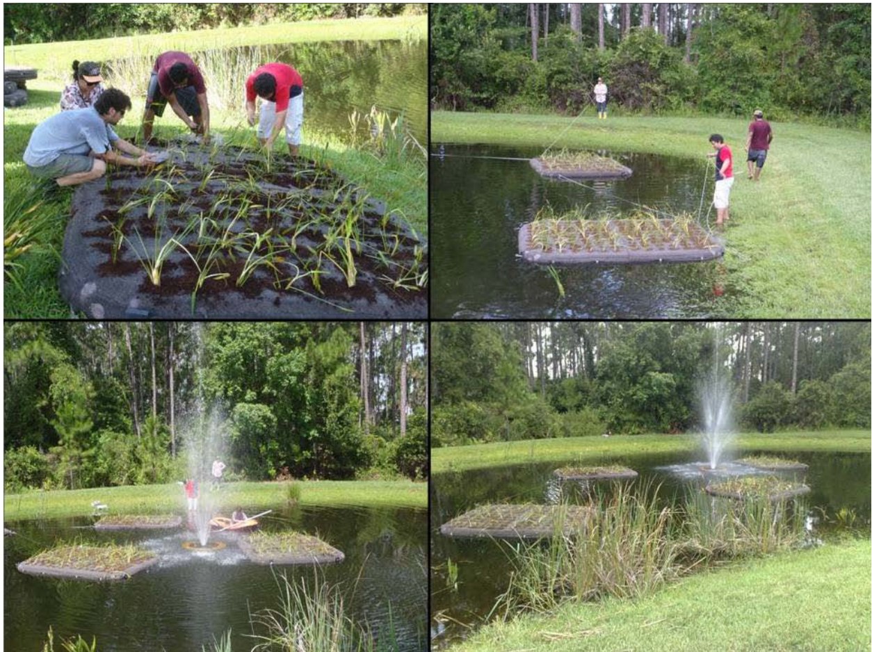
Figure 38: Deployment of floating wetland (7/15/2011)
