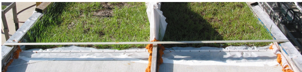
Figure 5. Perforated PVC pipe used for influent collection.
