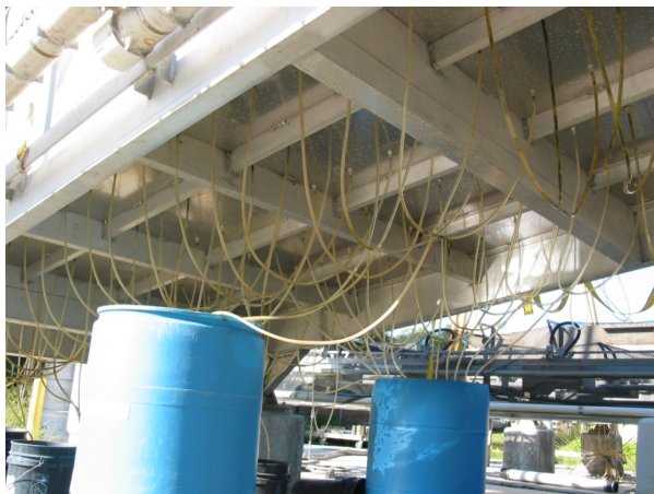
Figure 6. Effluent collection system.
