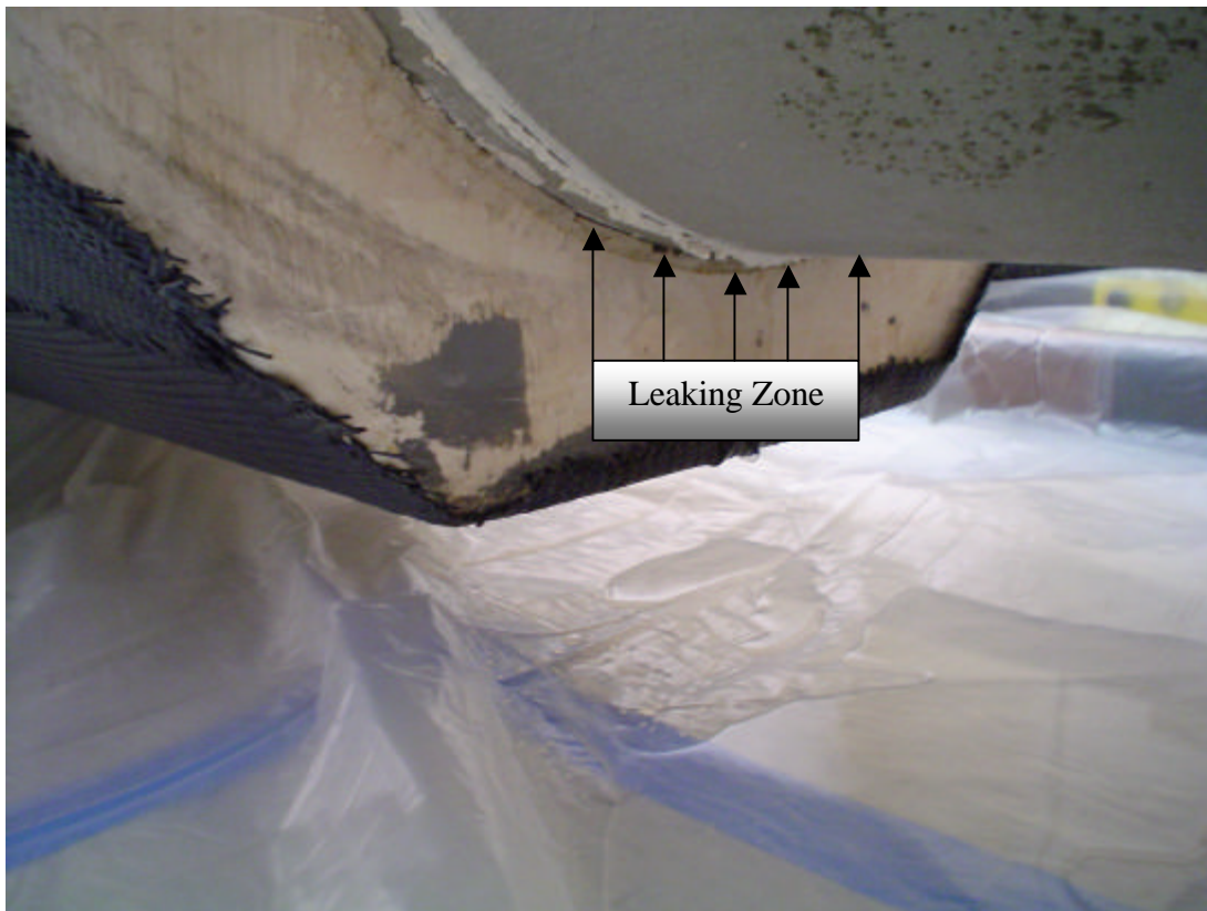
Figure 34: The Leak Emerges from the Interface in Between the Pipe and Hydro-stone
