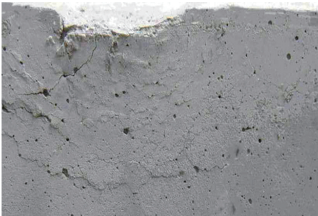
Figure 7 Compacted Damage Zone
