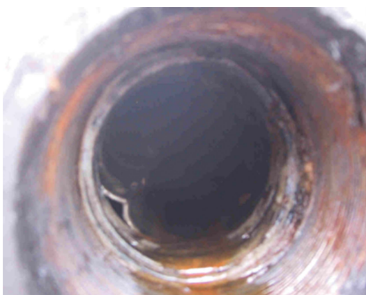
Figure 2 Internal Corrosion of Casing
