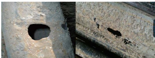
Figure 3 Casing Corrosion Punching
