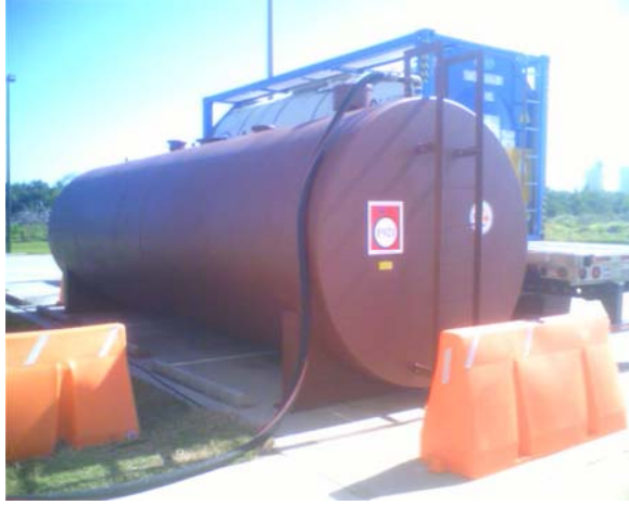
Figure 11. Double-walled 10,000gal isotank for Petroleum Storage
