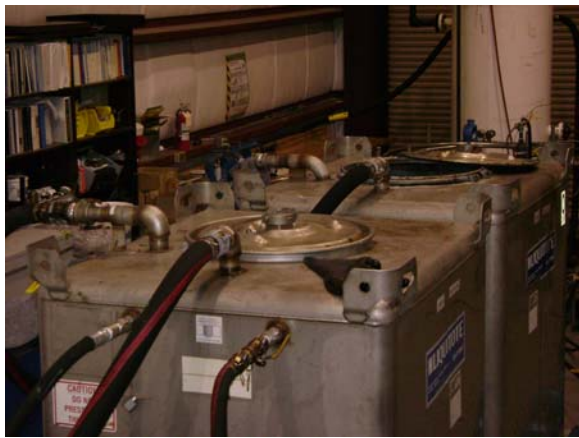
Figure 13. Stainless steel 550gal tanks with petroleum-rated hoses
