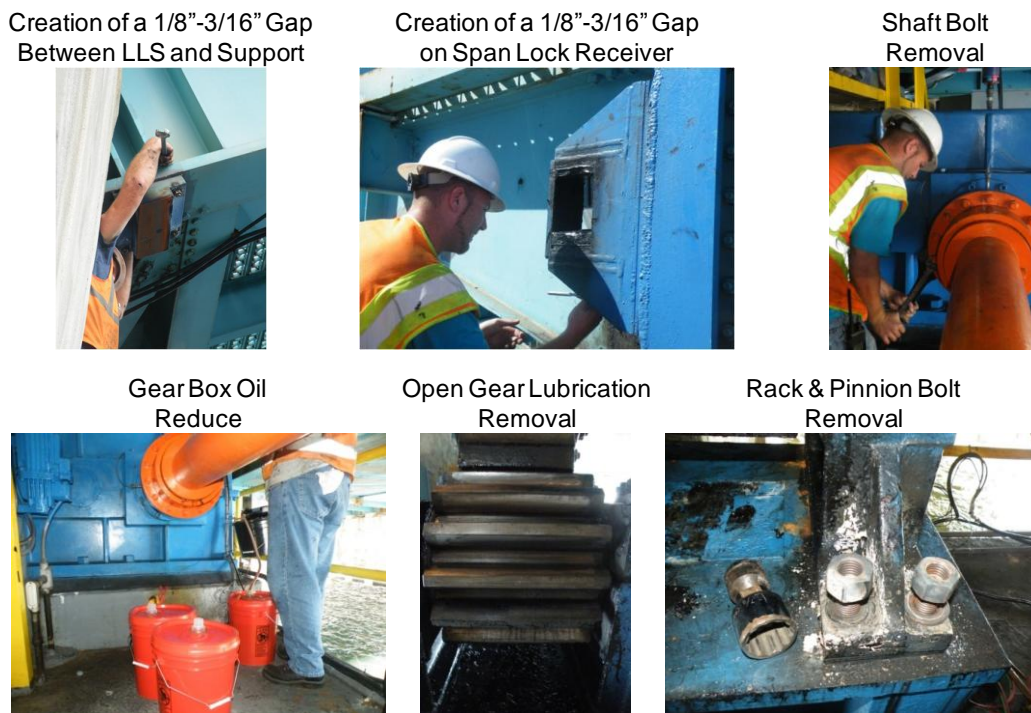
Figure 19: Damage tests on Sunrise Boulevard Bridge
