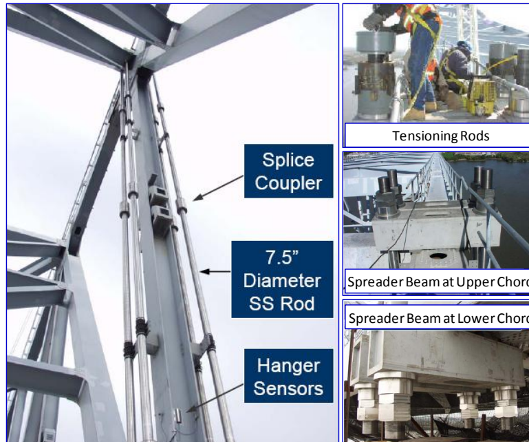
Figure 82: Retrofitted hanger and auxiliary system photos and drawings (Catbas et al. (2003) and photo credit to Dr. Kirk Grimmelman)
