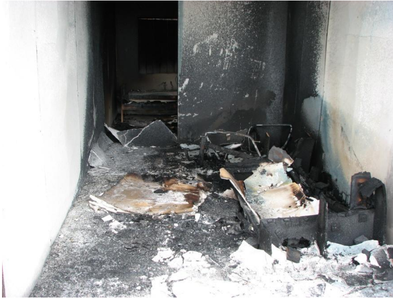
Figure 77: Container 8 Front Room Post Burn
