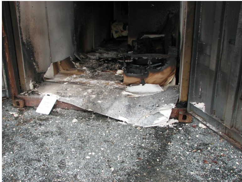
Figure 73: Container 7 Fallen Ceiling Post Burn
