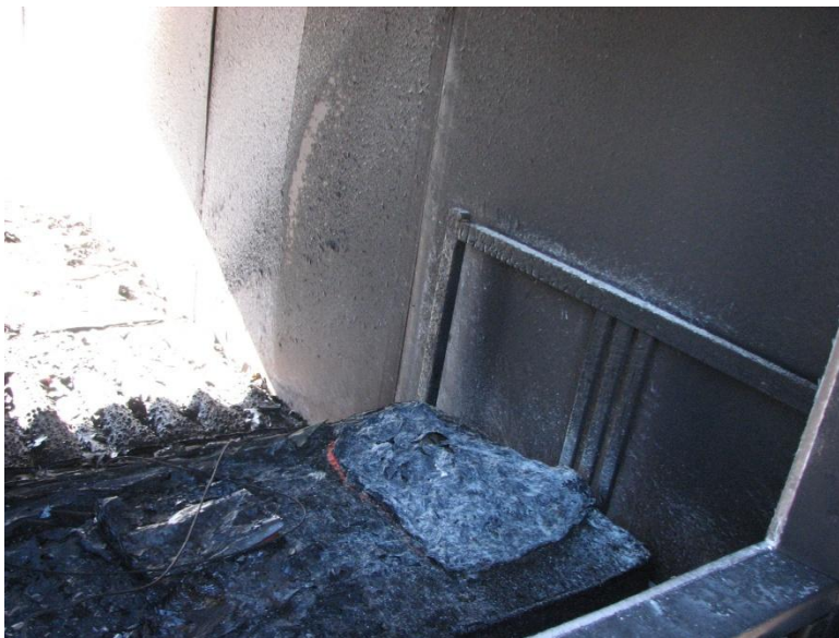
Figure 93: Container 11 Back Room Post Burn
