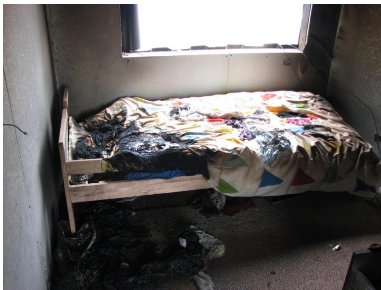
Figure 63: Container 5 Back Room Post-Burn
