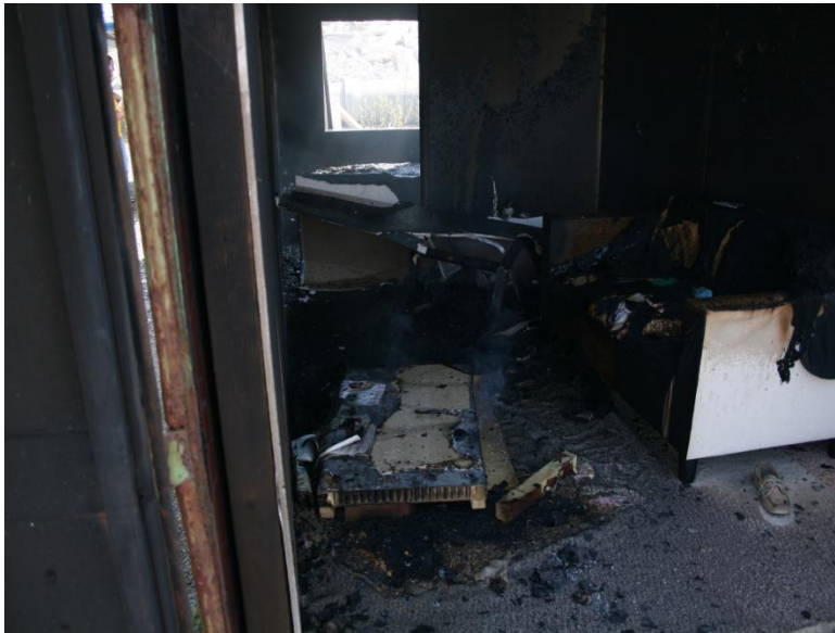
Figure 71: Container 6 Front Room Post Burn
