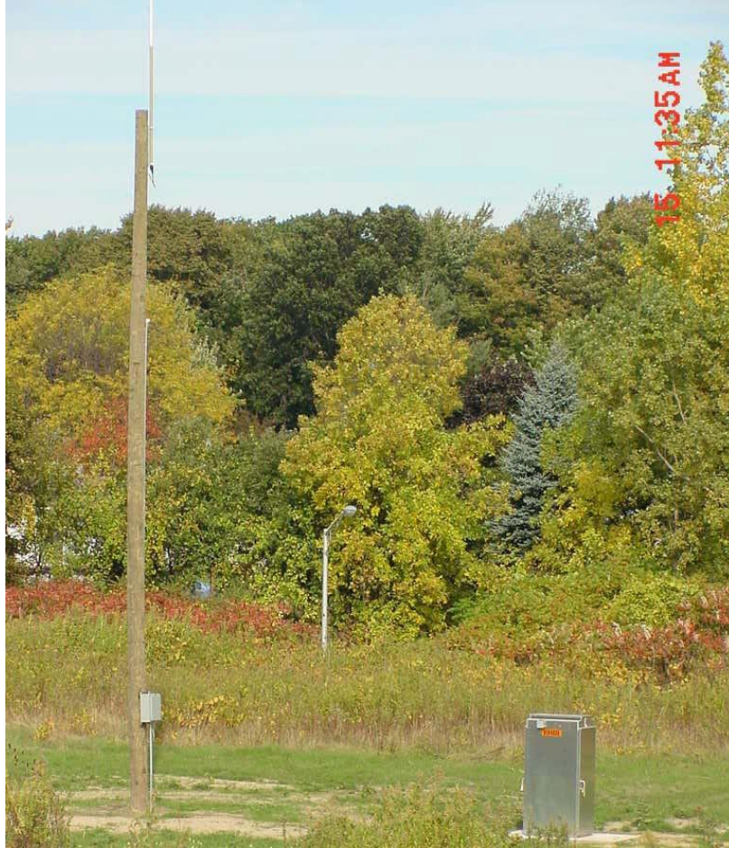
FIGURE 4 HAR STATION ALONG FREEWAY (NEUDORFF ET AL., 2003)
