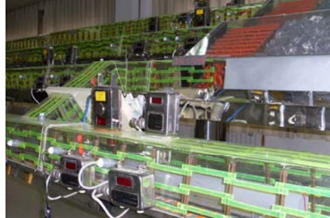
Fig. 8: Temperature sensor for test
