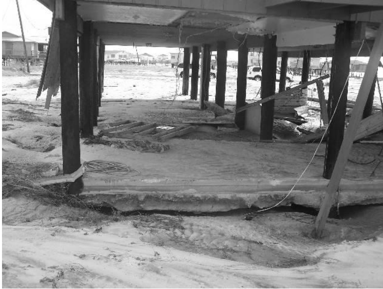
Figure 4 Scour occurring below Ground floor during hurricane Katrina (NIST-1476, 2006)
