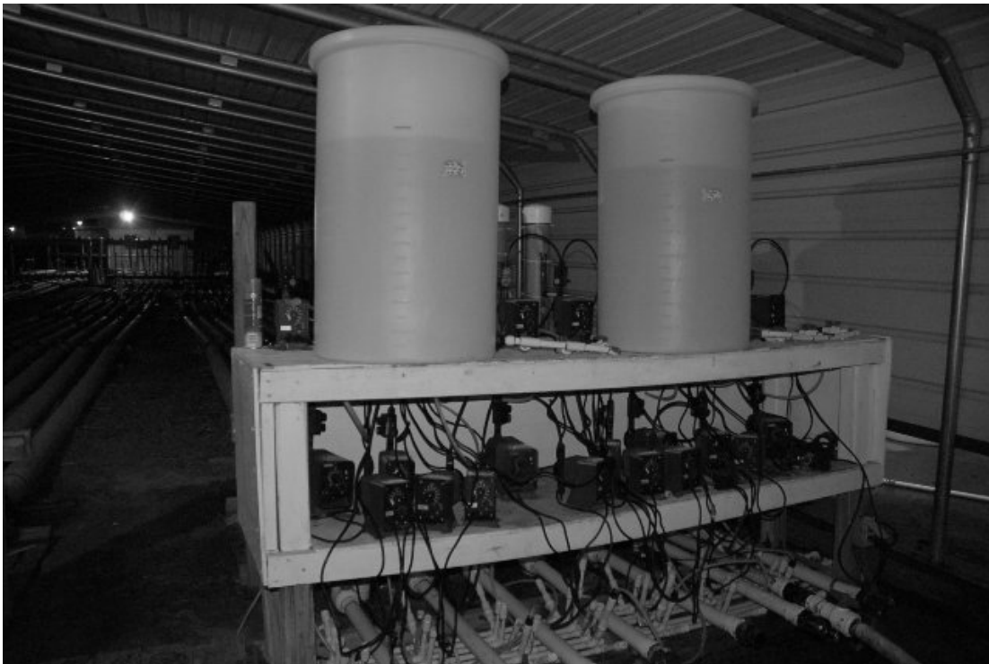
Figure 6.2 Corrosion Inhibitor Tanks and Feeding System
