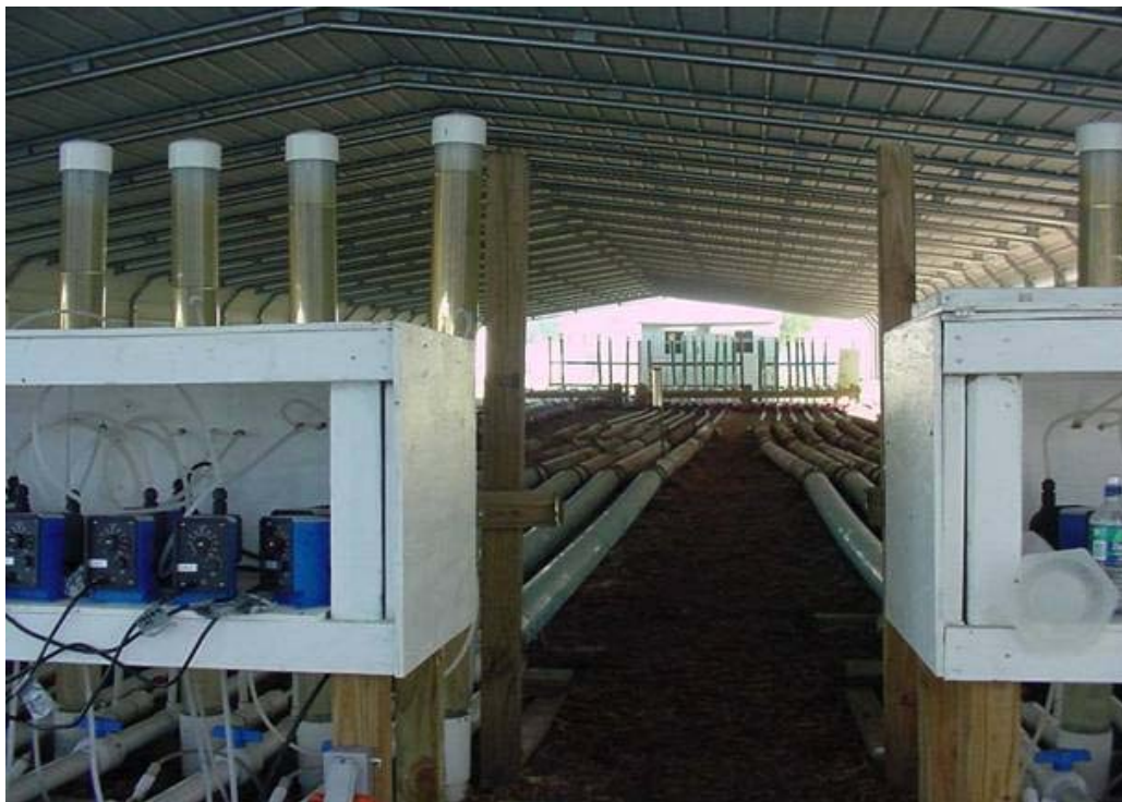
Figure 5.3 Influent Standpipes and Feed Pumps
