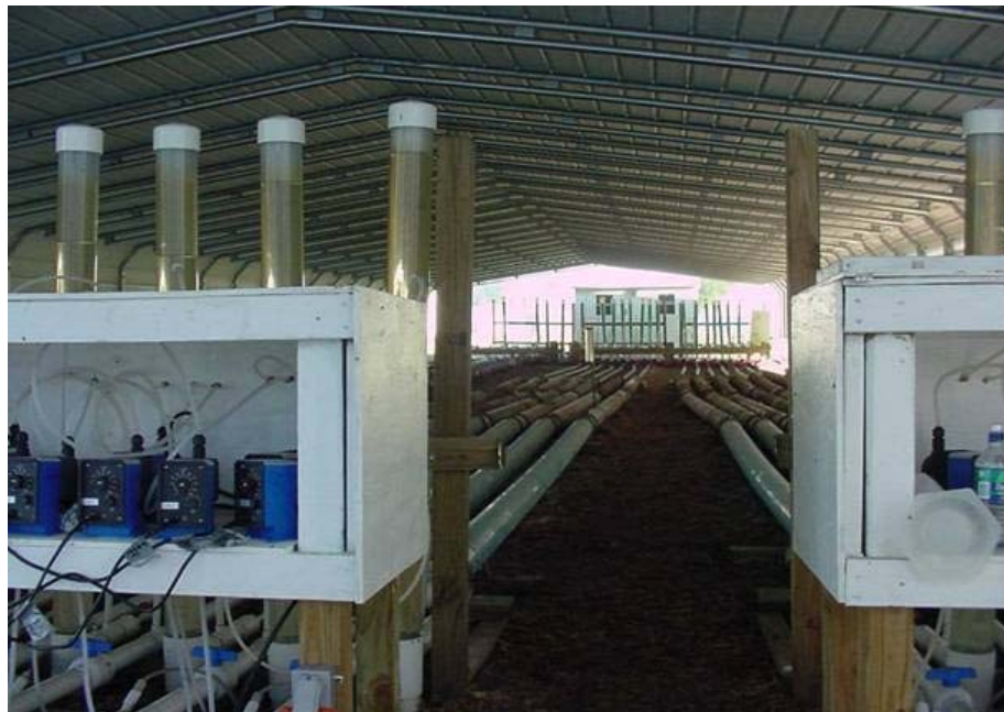
Figure 4.2 Feed Pumps and Influent Standpipes
