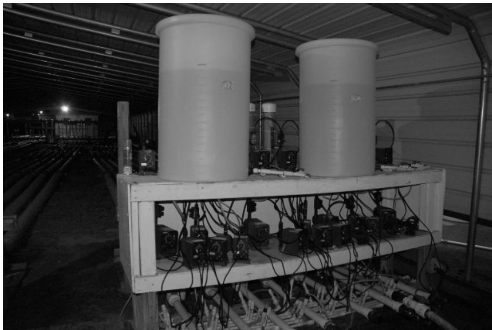
Figure 3.3 Corrosion Inhibitor Feeding System
