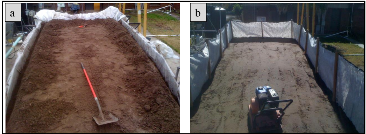
Figure 22 Silt fence installation on test-bed (a) 15 × 15 cm trench, and (b) BSRF silt fence installed
