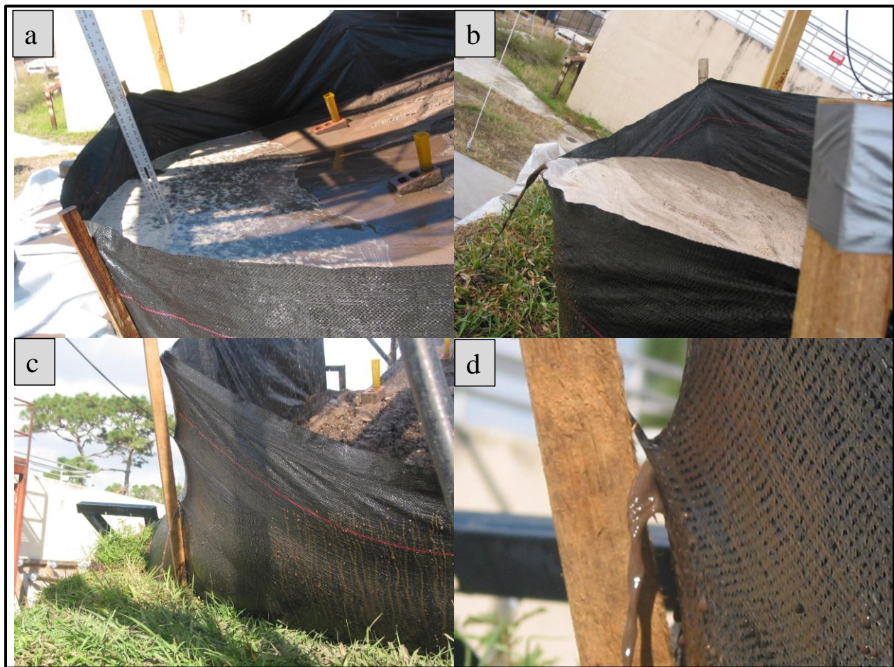
Figure 52 Effect of high backwater upstream of a silt fence: (a) flooding, (b) overtopping, (c) fabric ripped off the stake at the staple connection, and (d) larger fabric opening
