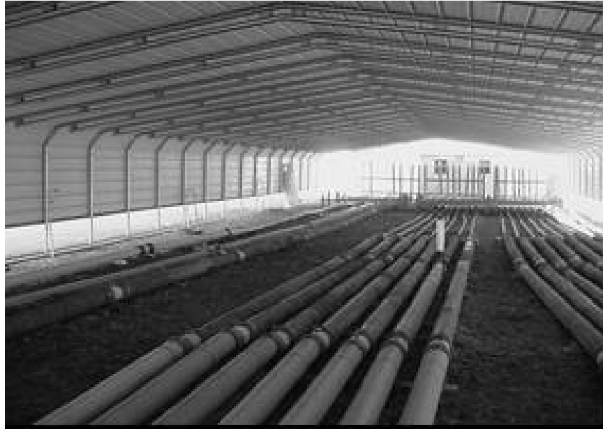
Photograph 6.1 Pilot Distribution Systems
