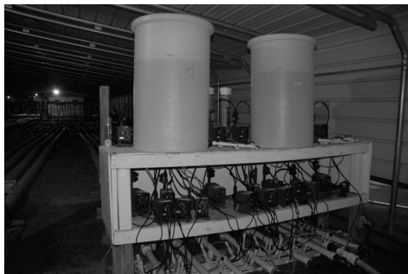
Figure 3.5 Inhibitor tanks and feed pumps
