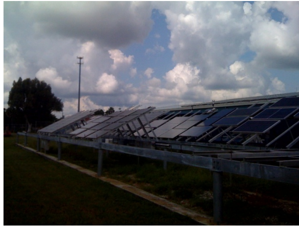
Figure 3-1 FSEC Outdoor Testing Facility
