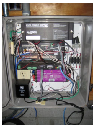
Figure 3-8 DAS at MMS System
