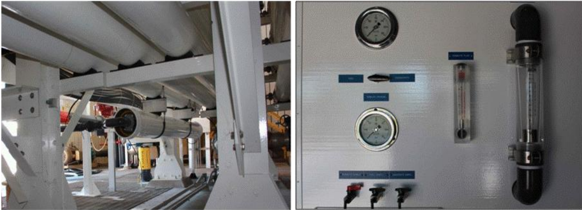
Figure 4-2: As Installed “Canary” Unit (left) and Instrumentation Panel (right)
