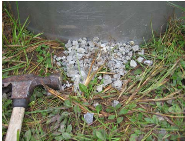
Figure 13: Plugged leaks around the buffer cylinder with Bentonite
